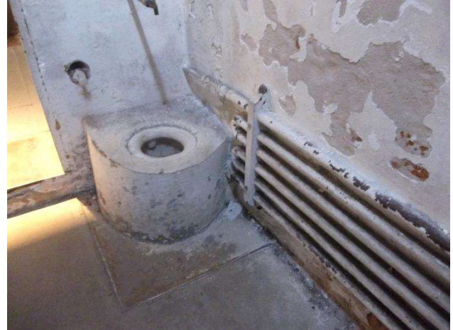
Each cell had a toilet with running water. Heat was provided by the pipes on the wall.
